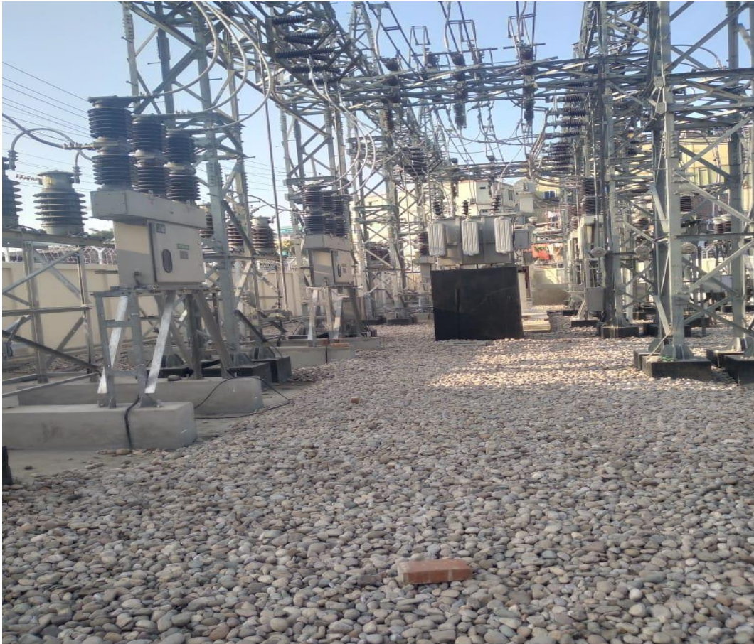
Figure: neat And Clean Workspace At Kalurghat SS
