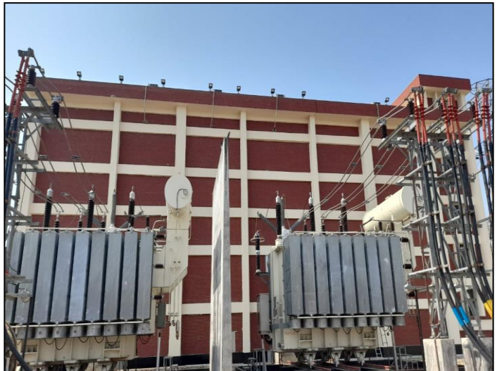
Fig-4: Transformer & GIS building of newly energized Madunaghat SS
