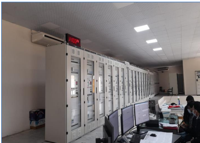
Pic-5: CRP of newly energized Madunaghat SS
