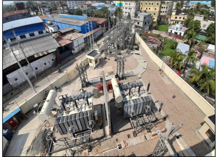
Fig-10: Transformer at Kalurghat SS
