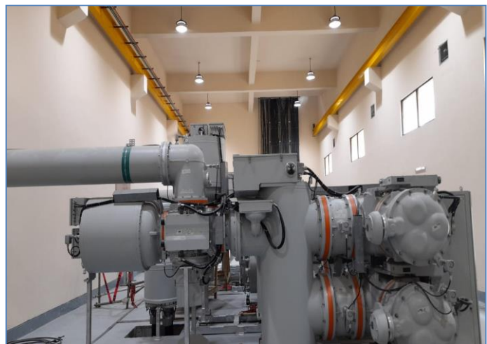
Fig-12: GIS at Kalurghat SS
