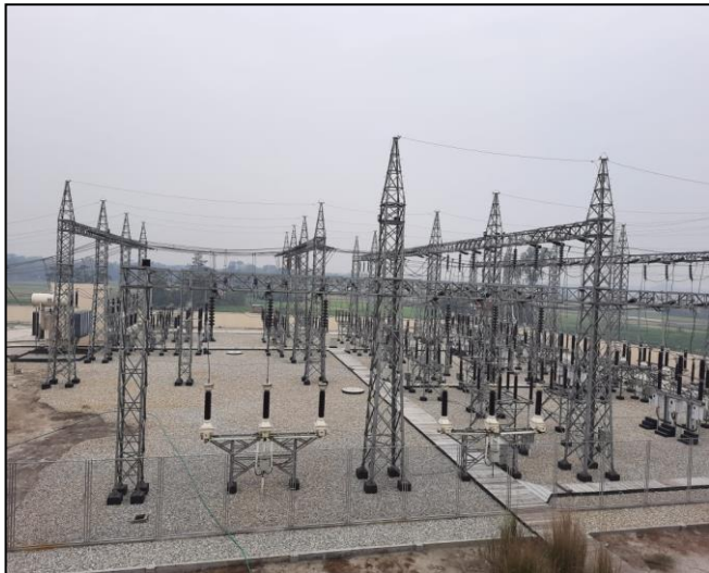
Fig-3: Switchyard of Newly energized Kachua AIS ss
