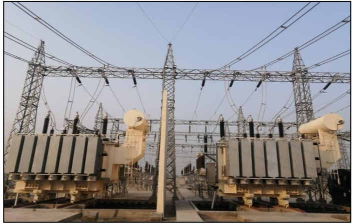
Fig-2: Transformer of newly energized Kachua AIS ss
