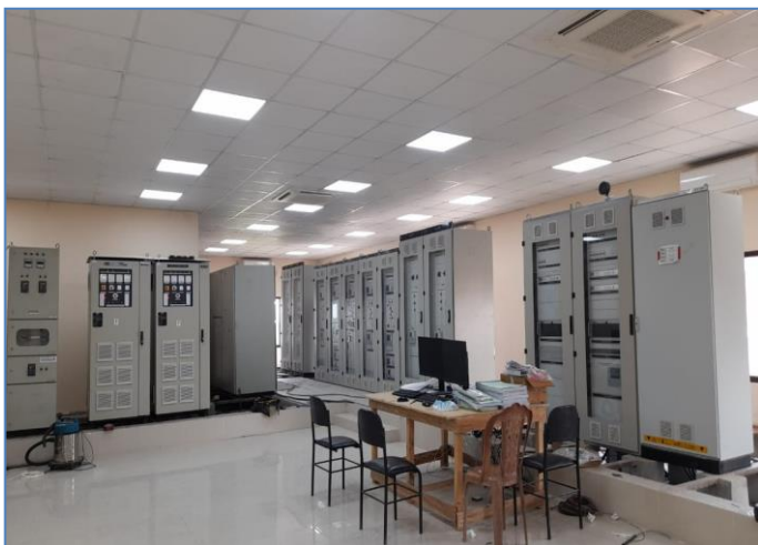
Fig-11: CRP at Kalurghat SS
